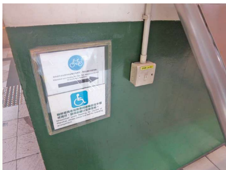
渡輪碼頭內的求助電鈴 Call bell at ferry pier
